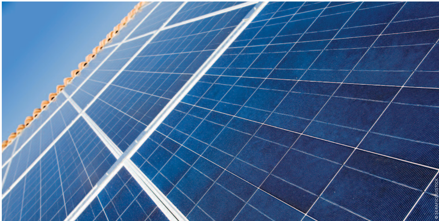
image PHOTOVOLTAIC PANELS ON A ROOF.
